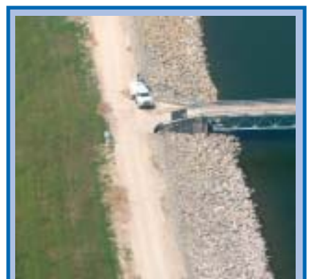
On the cover: The repair to the rip rap on Lake Livingston Dam is substantially complete 52 days ahead of schedule. The lake will now be allowed to return to the normal pool level of 131 mean feet above sea level as sufficient rain falls in the Trinity River basin upstream from the dam. Read more in the General Manager's column on page 4.
