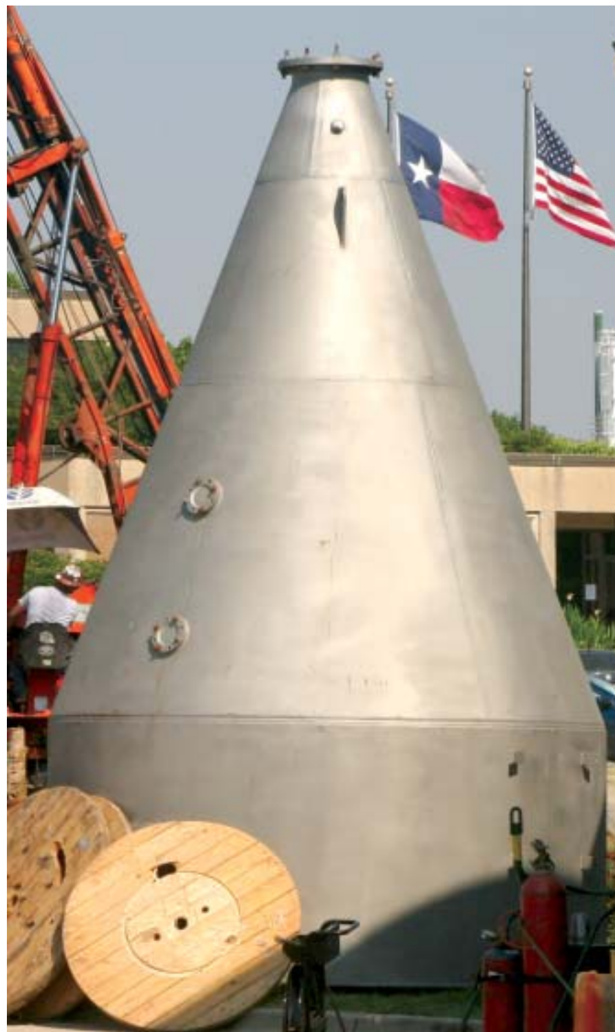
One of Two Speece Cones to be installed at CRWS this summer. Superoxygenation technology utilizes a reactor, such as a Speece Cone, to maximize oxygen absorption in wastewater, which eliminates most of the odor. The process is simple, does not use chemicals and has no moving parts other than standard wastewater pumps.
