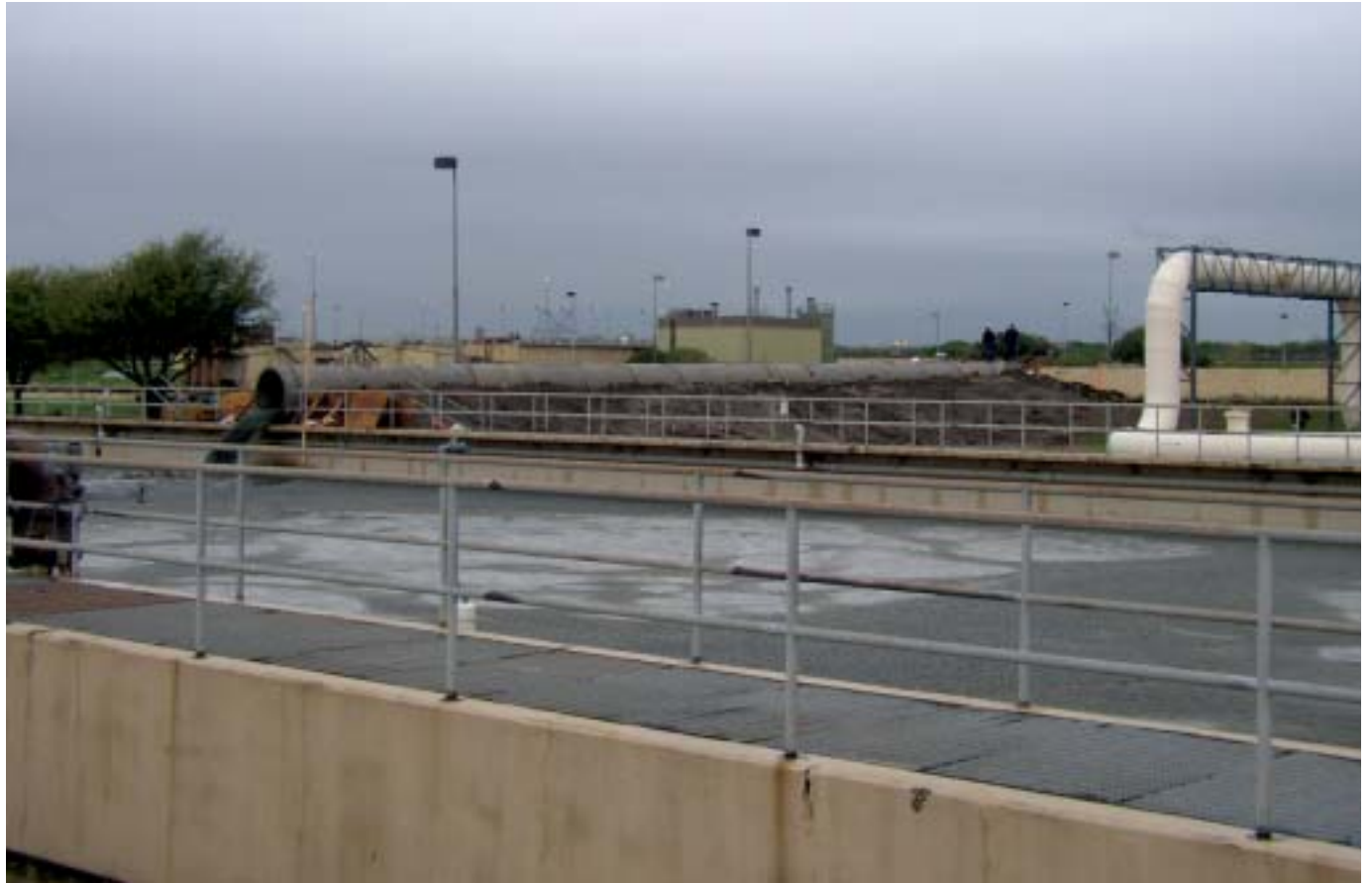
An earthen berm cradles the 140-foot long, 60-inch diameter pipe that transports rain-swelled wastewater from a moth-balled Primary Clarifier basin to an aeration basin at the CRWS plant. The pipe was installed to temporarily provide additional capacity while half of the plant was shut down for repairs. Installation of the pipe was complete shortly before a weekend of record-setting rainfall at the plant and surrounding cities.
